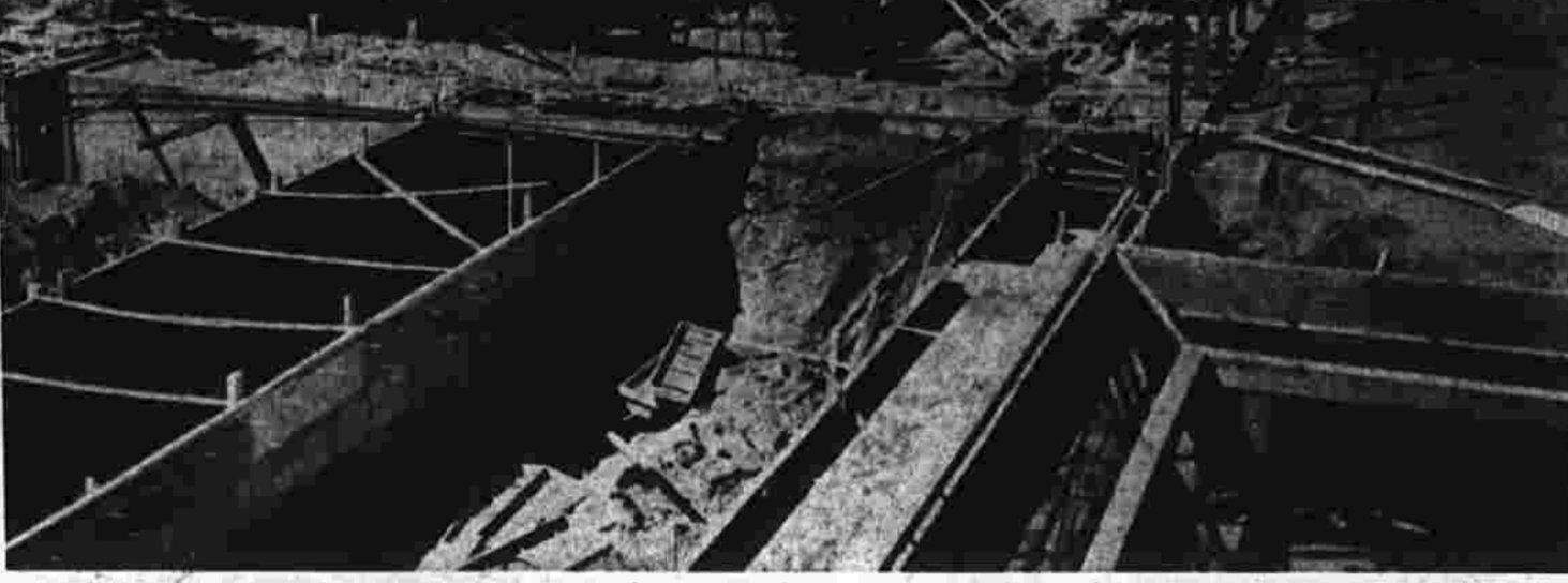
Flat and sketched in bold outline only a few weeks back, the new Manchester High School begins to take on its vertical dimension as work by the M. S. Kothler Co. contractors continues...
